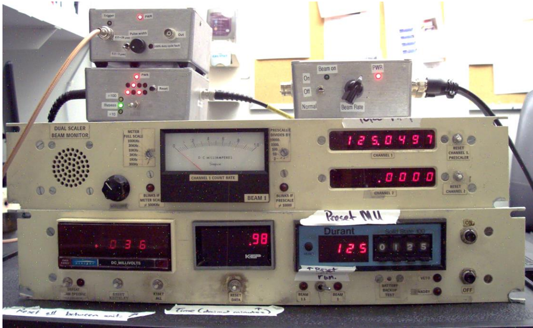
Dosimetry control unit from HCL at MGH with additions
