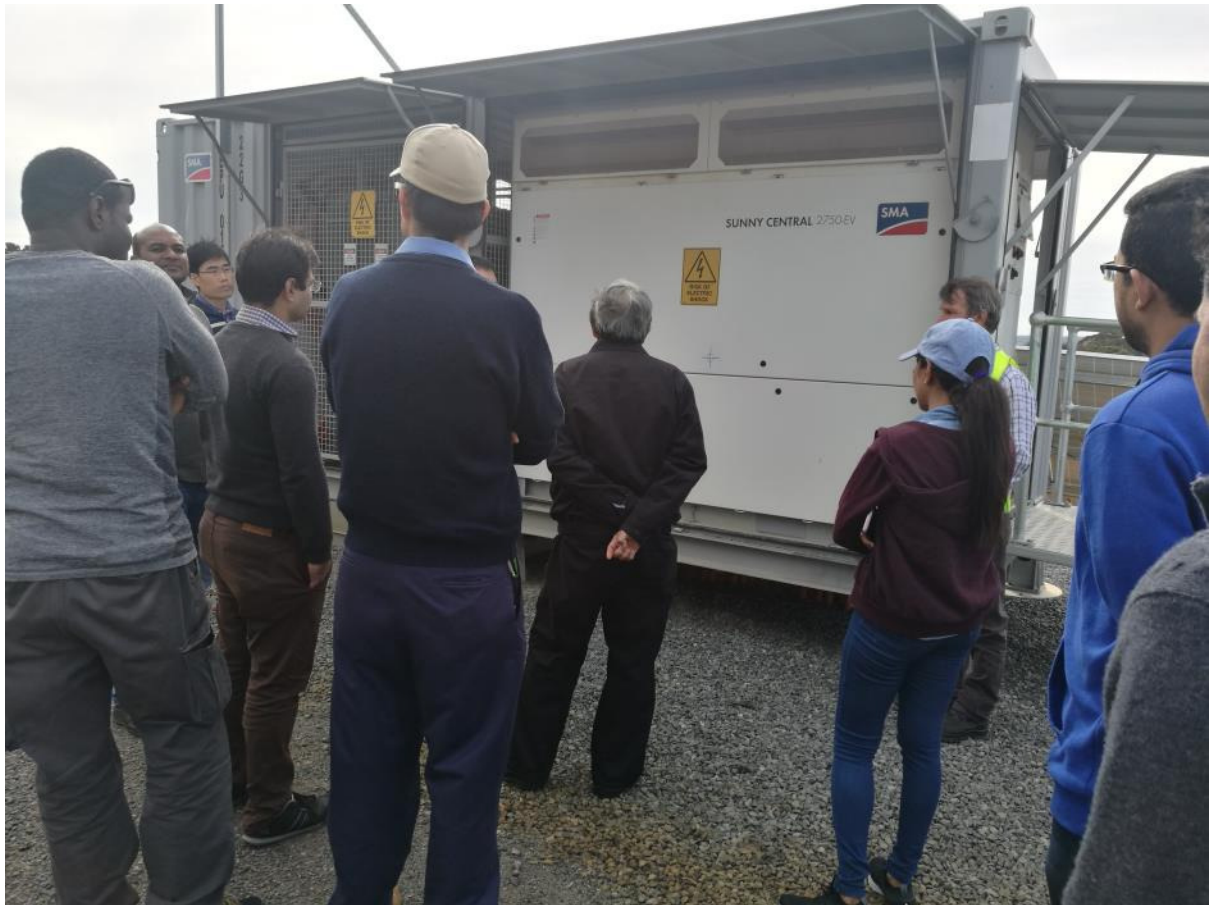
Photograph: Students watching the solar inverter and transformer local substation at the solar farm.
